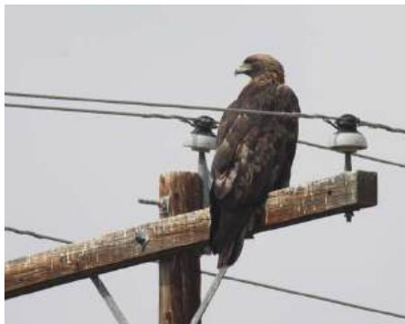
▲ A golden eagle sits on an unprotected pole, which needs a conductor cover added.
