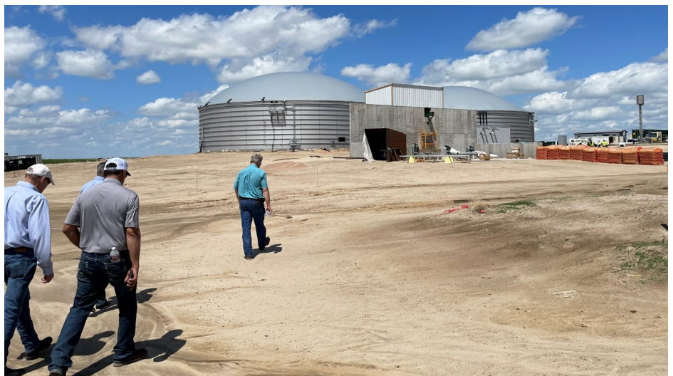
Dairy farmer Chris Kraft, far right, leads a tour in May 2023 of the anaerobic digester under construction at his Quail Ridge Dairy near Fort Morgan. Photo courtesy of Morgan County REA.
