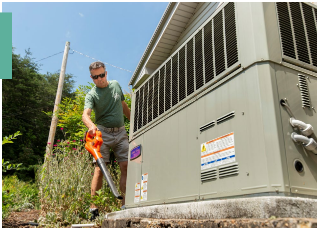
◀ The lifespan of a heating and cooling system ranges from 15 to 20 years. Proper maintenance and lower use can increase the life of the equipment. Photo source: Mark Gilliland, Pioneer Utility Resources.
