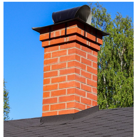
▲ The metal flashing between the roof and chimney should have a water-tight seal. If the flashing is badly rusted, replace it.
